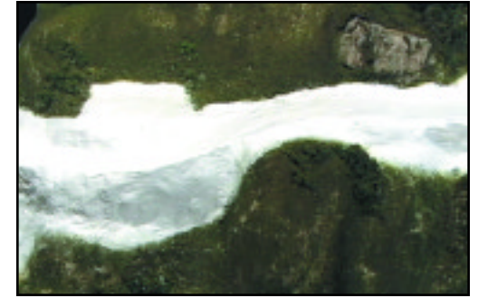
Cover Risers with a new layer of Plaster Cloth and blend this into the existing hardshell.
