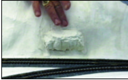
Test fit rock outcroppings before adhering them in place with Lightweight Hydrocal.
